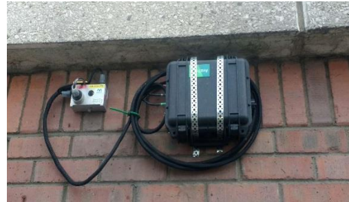
Photo 9.1: Typical Vibrograph installation
